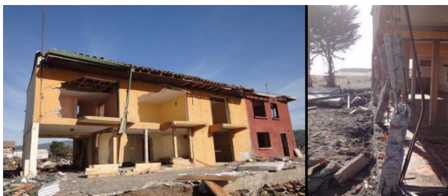
Figure 1 Global (Left) and Local (Right) Structural Damage
