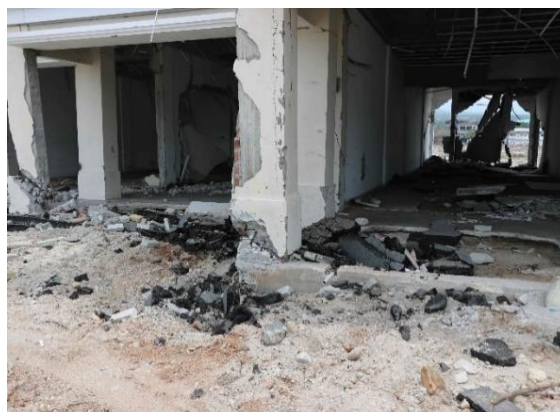
Figure 2 Concrete Debris Impacts
