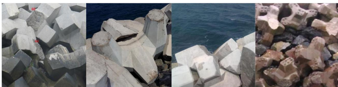
Figure 1 Broken Single Layer Units in Reality
