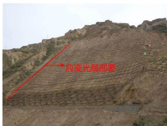
Figure 5 Deployment Position of the Strain-sensing Optical Cable
